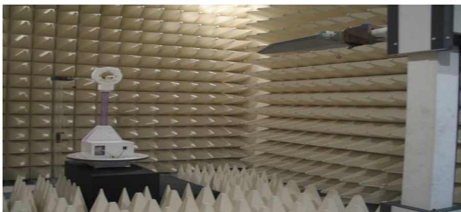
Figure2. Photograph of 3m Fully-Anechoic Chamber
