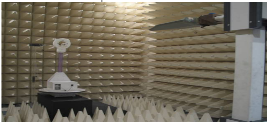
Figure2. Photograph of 3m Fully-Anechoic Chamber
