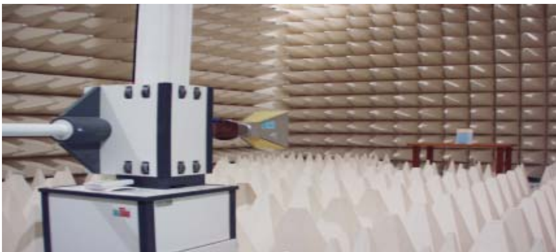
Figure2. Photograph of 3m Fully Anechoic Chamber
