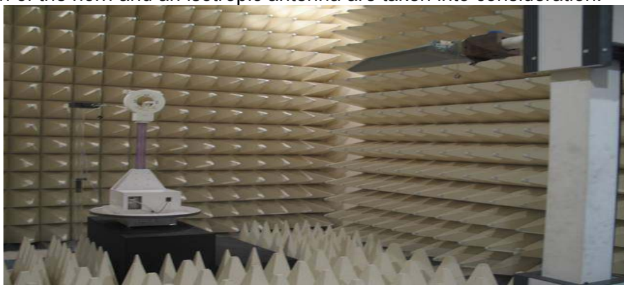
Figure2. Photograph of 3m Fully-Anechoic Chamber
