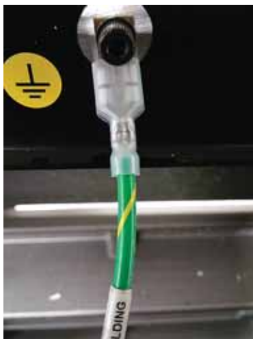
Figure 4-118 Ground wire connected to panel
