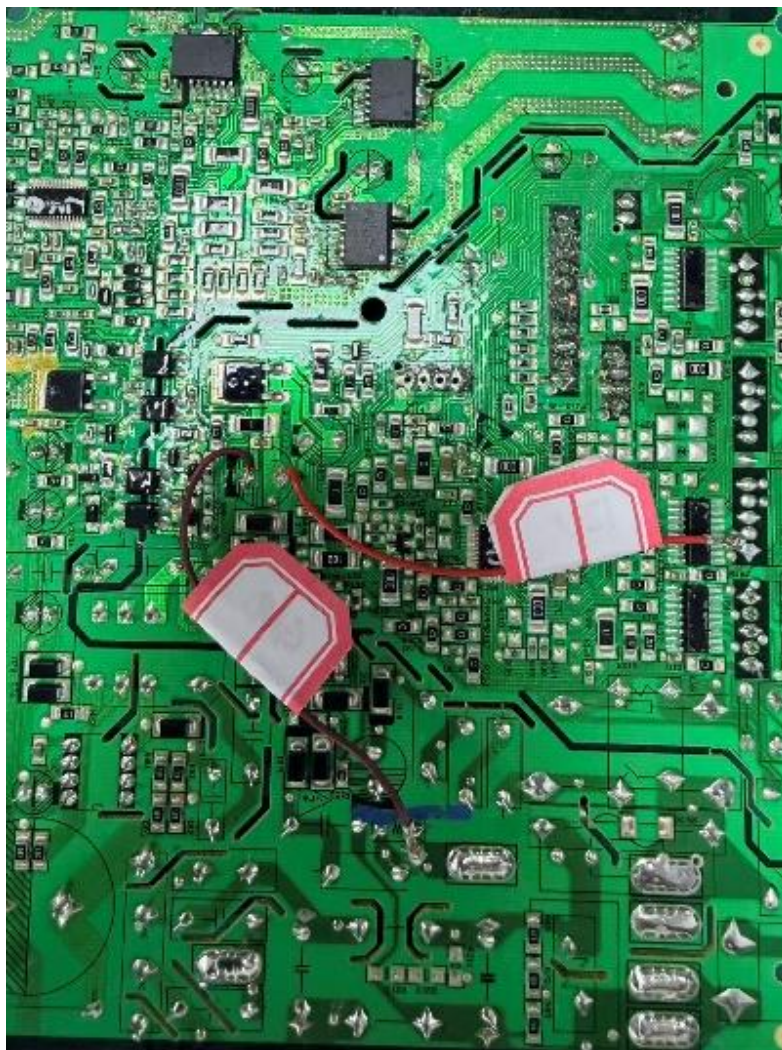
Figure 5: Electronic Control Board Power Supply Wiring
